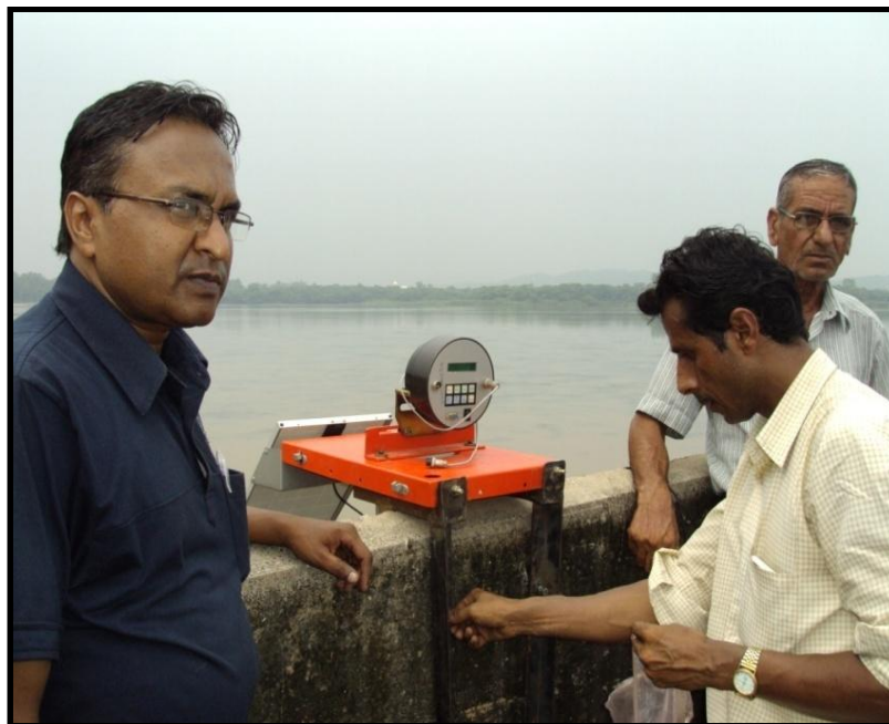
Fig. 31: Automatic water level recorder installed at the lake
